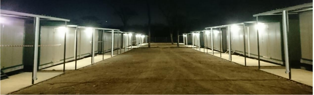
Figure 2. Montepuez Graphite Project: View of permanent camp showing night commissioning of electrical fit out.
