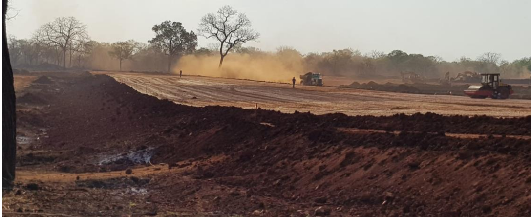
Figure 4. Montepuez Graphite Project TSF civils work, managing moisture content to ensure appropriate compaction and wall strength are progressing well.
