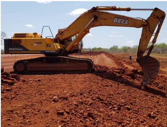
Figure 5. Montepuez Graphite Project TSF wall progressing well with excavator forming final wall angles
